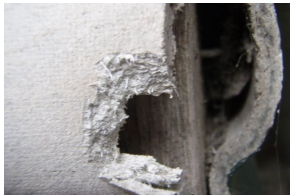
ACM or Asbestos Sheeting
