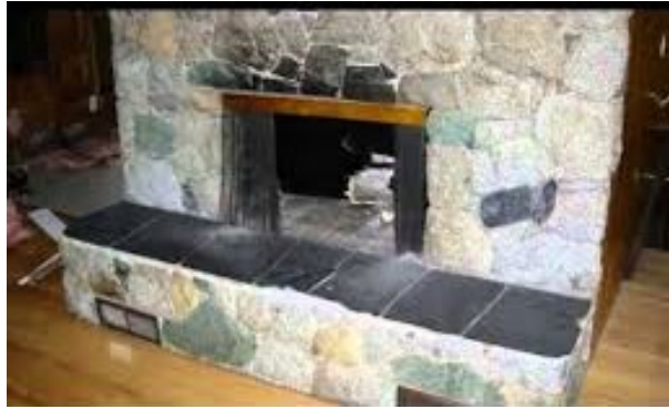
Figure 2 Insulation around wood heaters
