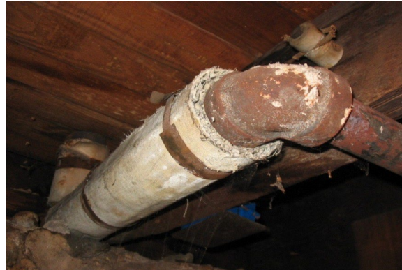
Asbestos used as insulation on pipes – lagging
