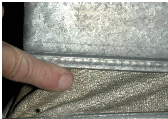
Figure 5 Asbestos cloth duct vibration dampener
