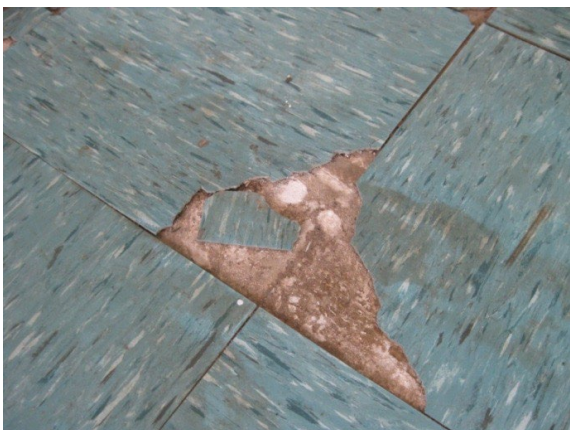
Damaged floor tiles containing asbestos
