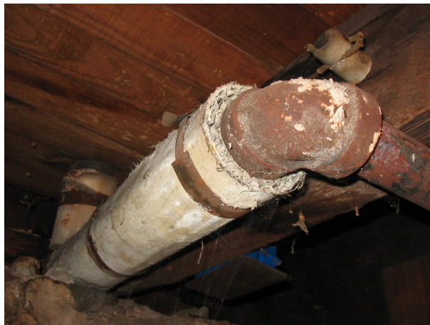
Figure 3 Thermal insulation for pipes and boilers
