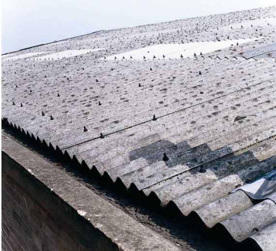
'Super 6' Asbestos Sheeting as a roofing material
