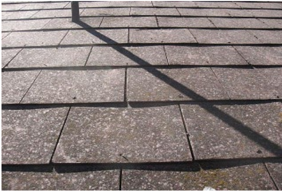
Asbestos Roof Tiles [an example of non-friable asbestos]
