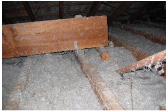
Asbestos fibre as ceiling insulation [an example of 'Mr Fluffy' friable asbestos]
