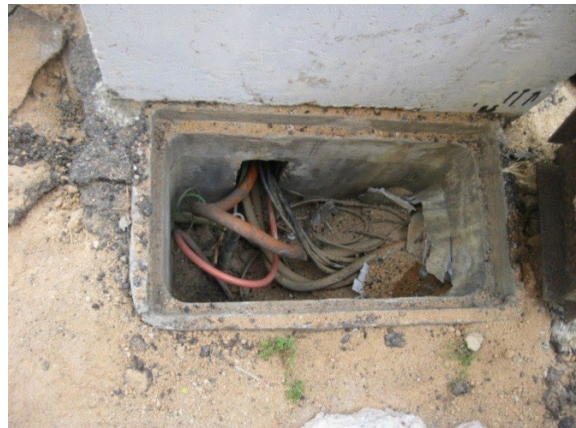
Asbestos Containing Material (ACM) in a telecommunications pit
